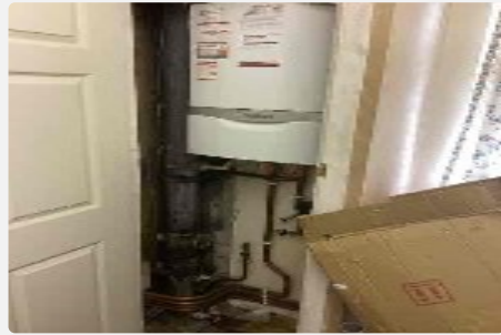
Gas boiler cupboard
