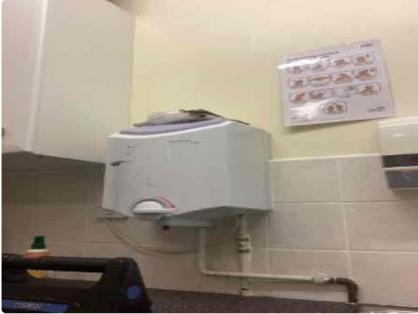
Disconnected water heater
