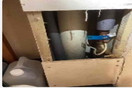
Incoming mains water supply
